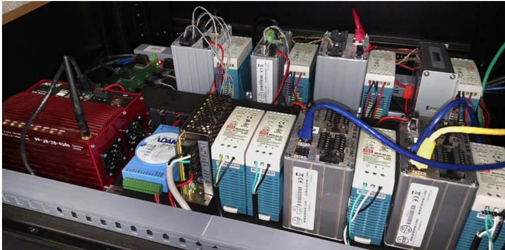
The Opto 22-based WindCapture system allows SCADA Solutions to quickly scale back power generation during periods of low demand.
