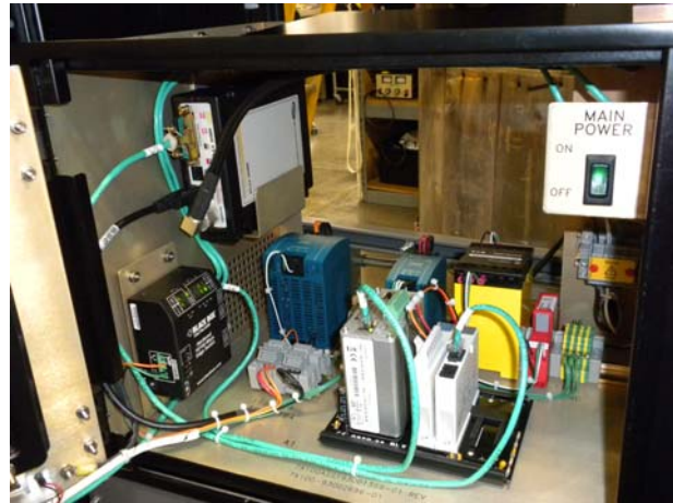
The RRCS, which comes with both wired and wireless connectivity and a touchscreen interface, is a new system that will be initiated at the Vero Beach Municipal Airport next year, followed by additional deployments at many other airports.
