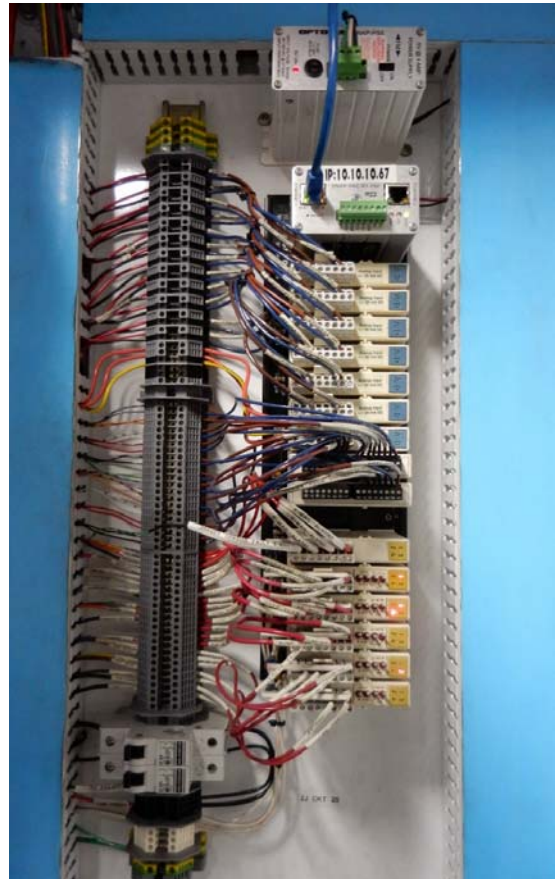
Some of the more than 1000 points of I/O the Toyo Tanso USA factory uses in their SNAP PAC control system.
