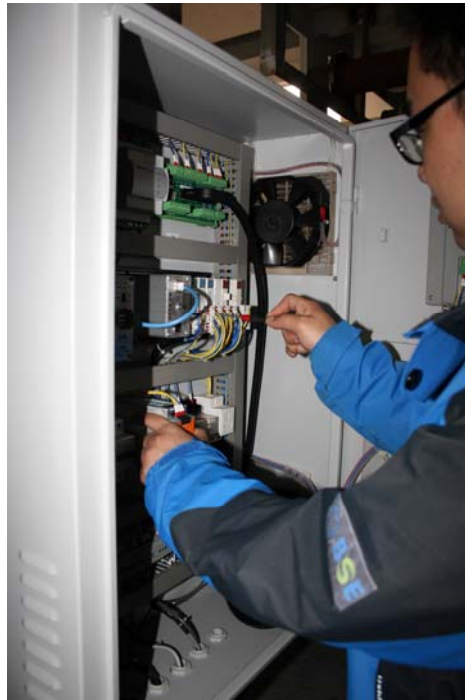
A BSE technician adjusts an Opto 22 SNAP PAC control system in a maglev chiller.
