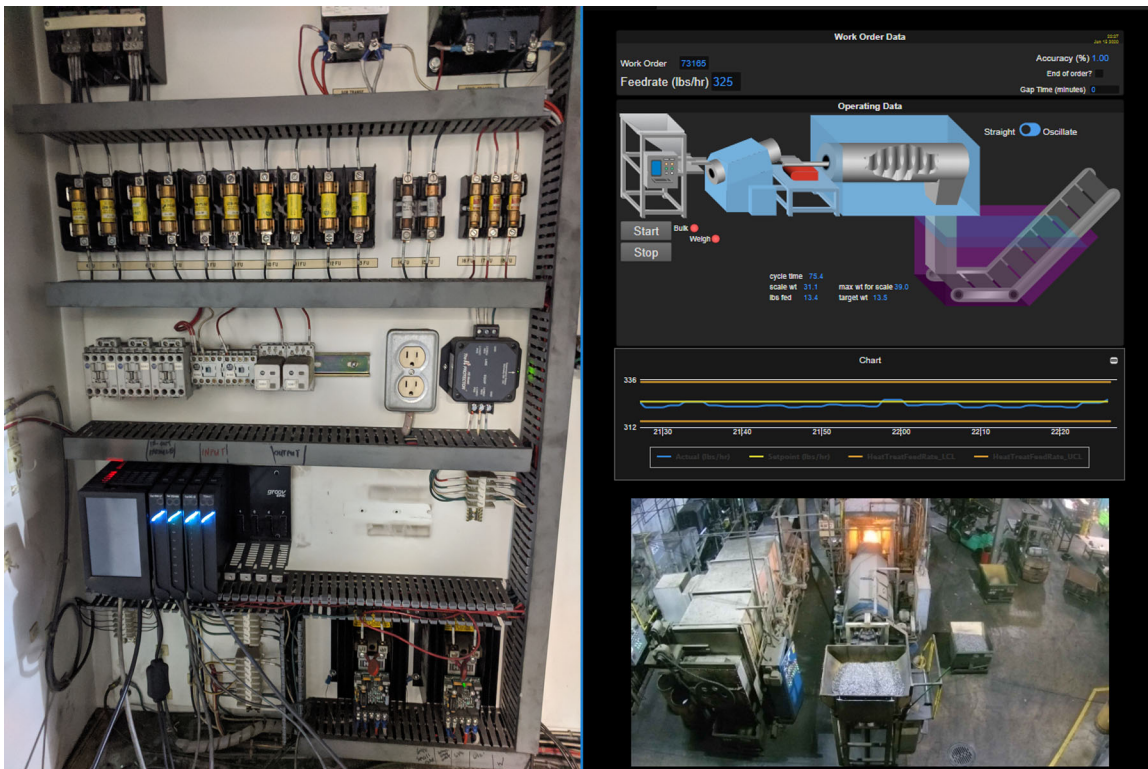
New electrical panel layout with groov EPIC and accompanying groov View HMI
