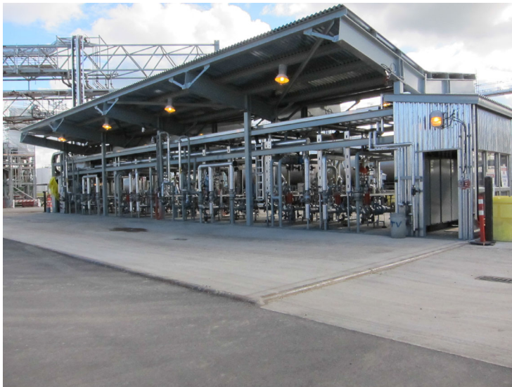
A loading rack for tanker truck transfers
