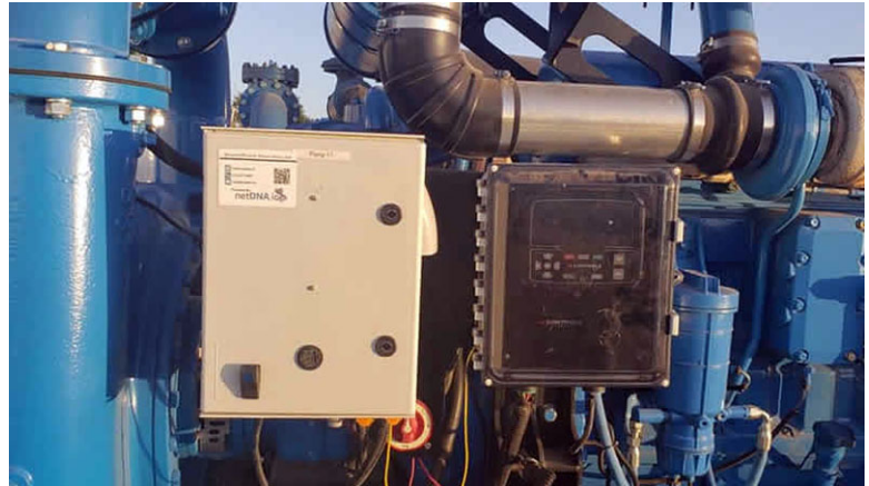
Pump and smart pump controller (side view)
